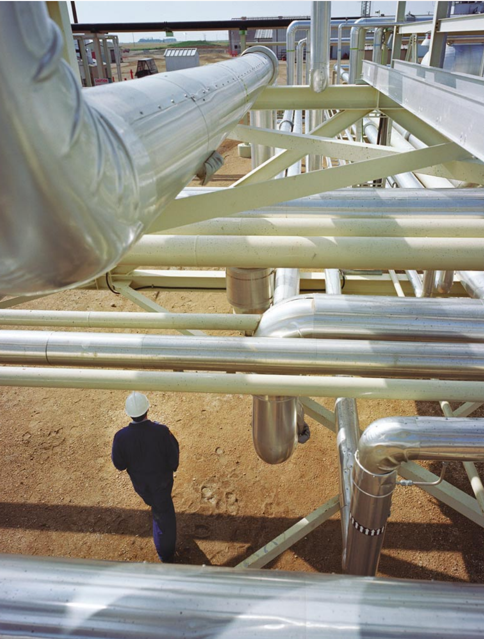
Above: Process piping in Weyburn Unit plant yard.
